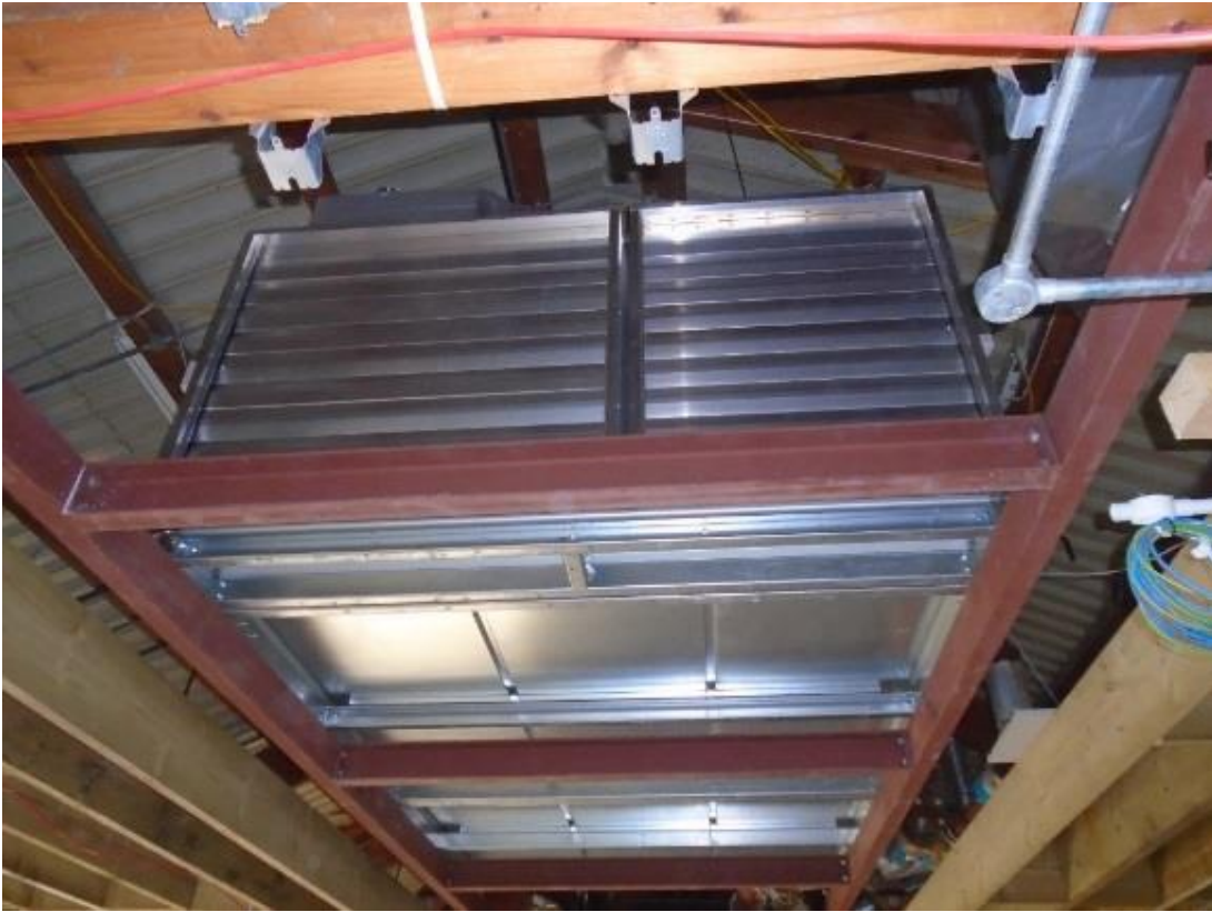
Coconut Grove air handling unit
